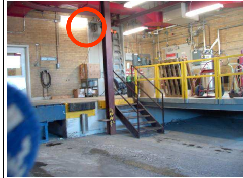
Indoor with sunlight, CCTV
